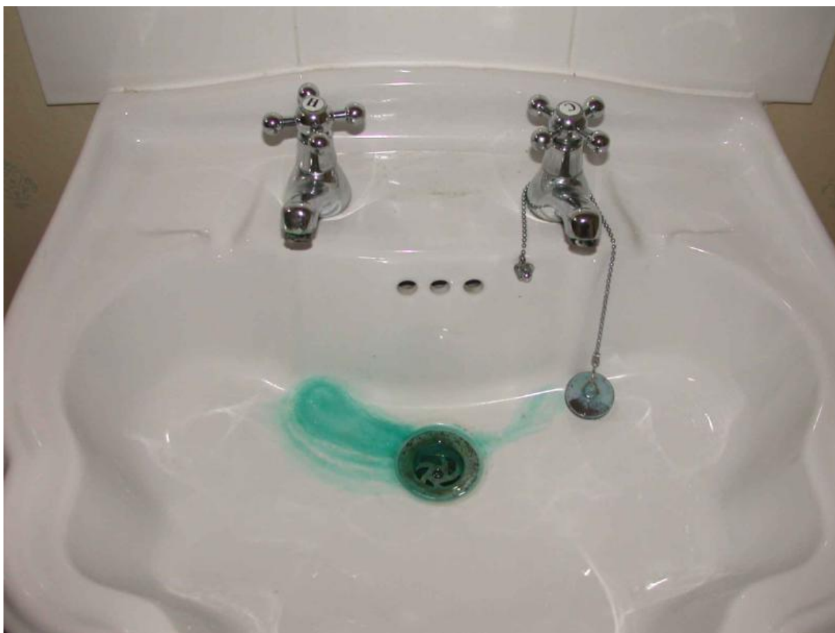
Figure 5b Staining in hand basin caused by blue water.
