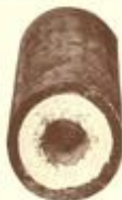
Not rust—but scale. It forms in any kind of pipe—iron, lead, or brass.
